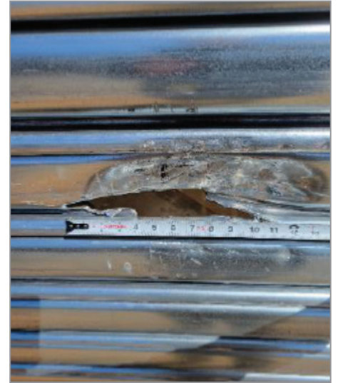
Specimen #3 Center of door, post attack 30 min entry time
